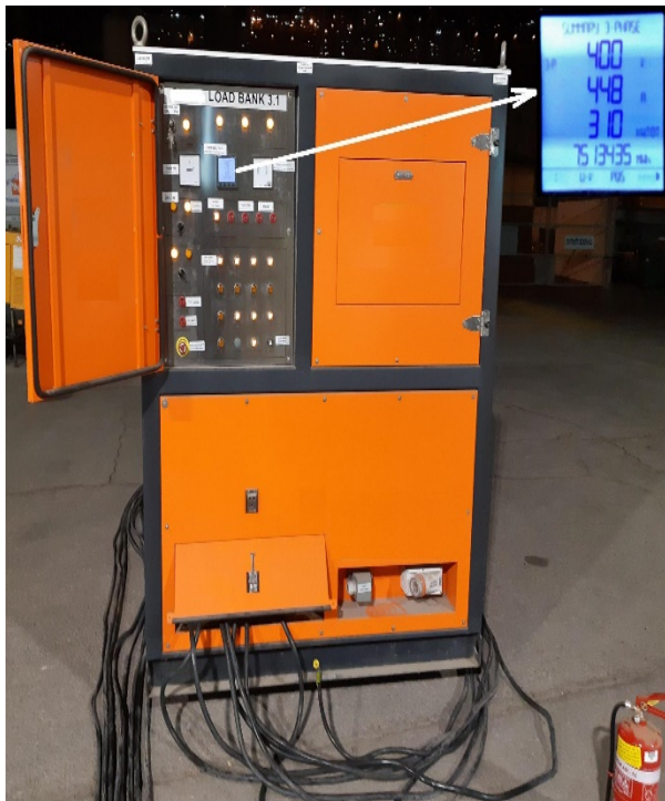
Fig. 11. Load resistance used during DG testing The controller display shows voltage (400V) and current (448A) parameters used during testing.
