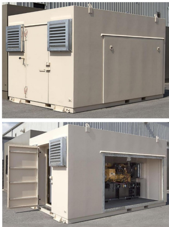
Fig. 14. Protective containers for immovable DGs. The vents are closed with honeycomb panels.
