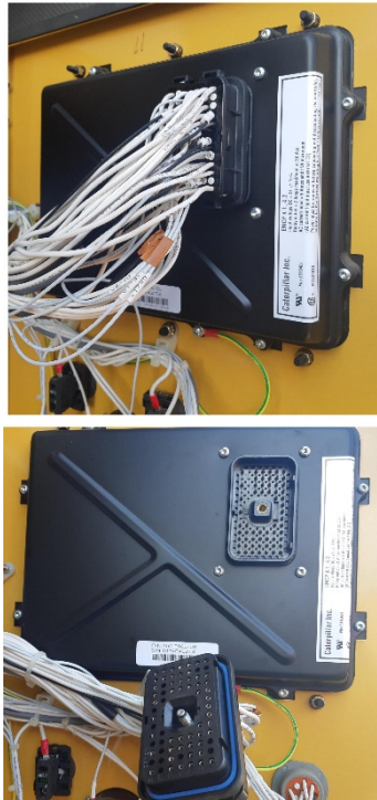
Fig. 7. Disconnection of cable harness from the main controller as protection from HEMP impact
