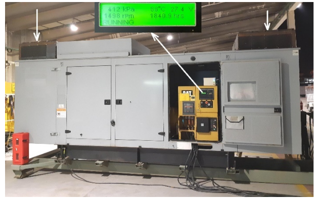
Fig. 12. DG with ventilation panels attached to it (shown by arrows) during testing. The controller's display shows an 88°C temperature, which corresponds to a full load of DG without additional ventilation panels. This temperature remained unchanged during testing.
