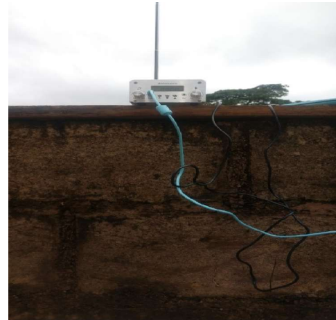
Figure 2: Pictorial representation of the transmitter mounted on the fence
