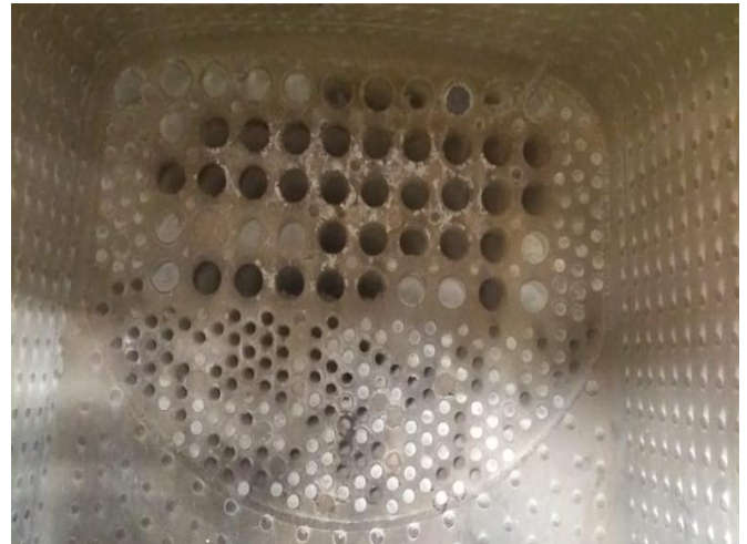
Figure 7: Blocked fire tubes of wood boiler due to ash deposits
