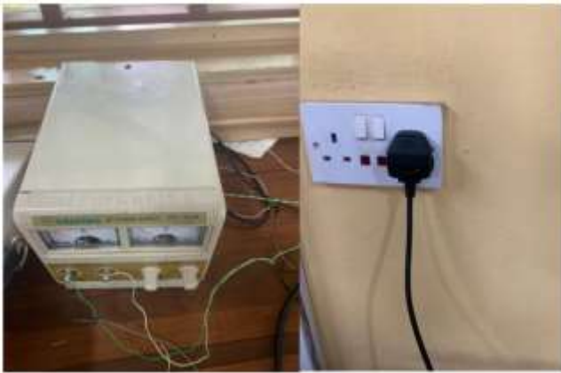
Figure 1: Power source used (12 V DC and 230 V AC)
