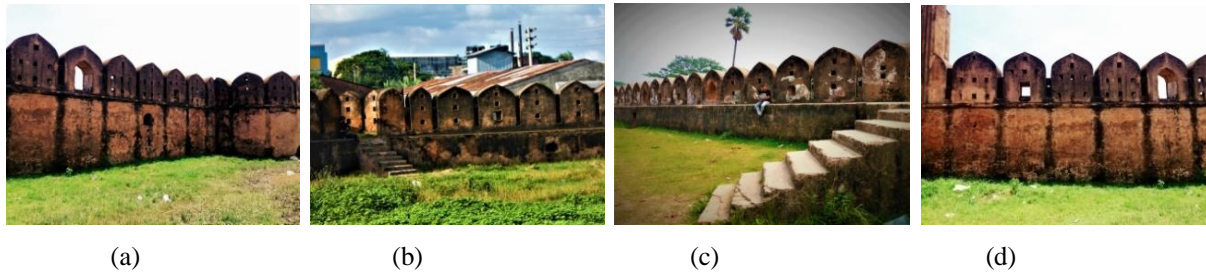
Figure 16 Shows:: (a),(b),(c),(d) Details of Ancient Khizirpur Fort (Presnet Hajiganj Fort) Defensive Wall Structure.
