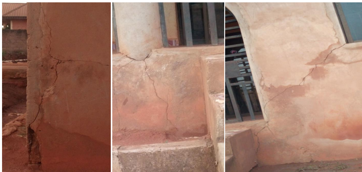
Figure 1b. Signs (cracks) of foundation failure observed on a nearby building.
