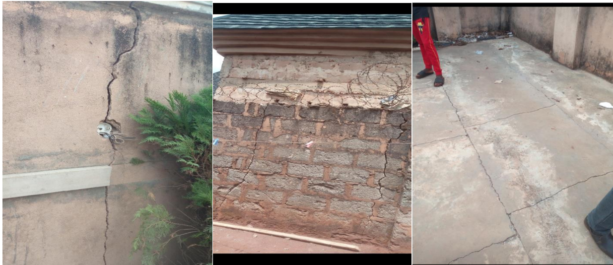
Figure 1a. Cracks on the main building of interest at the study location.
