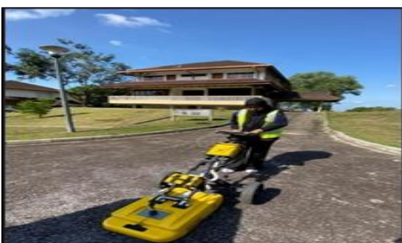
Fig. 3 Underground Utility Detection using IDS GPR Detector Duo metallic and non-metallic pipes and cables
