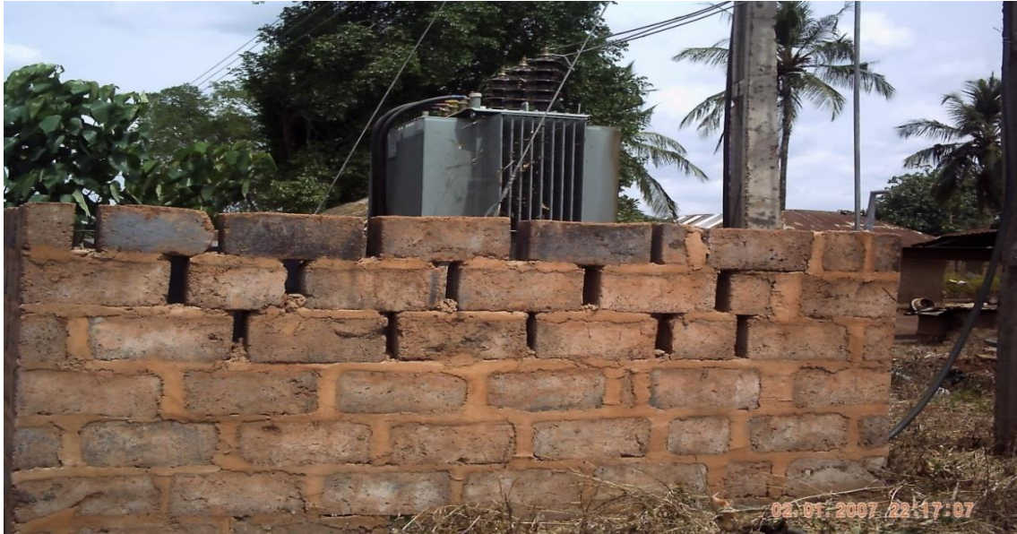
Plate 3: Electricity Transformer donated by a migrant to Jerico-Ugboju in Otukpo L.G.A of Benue State
