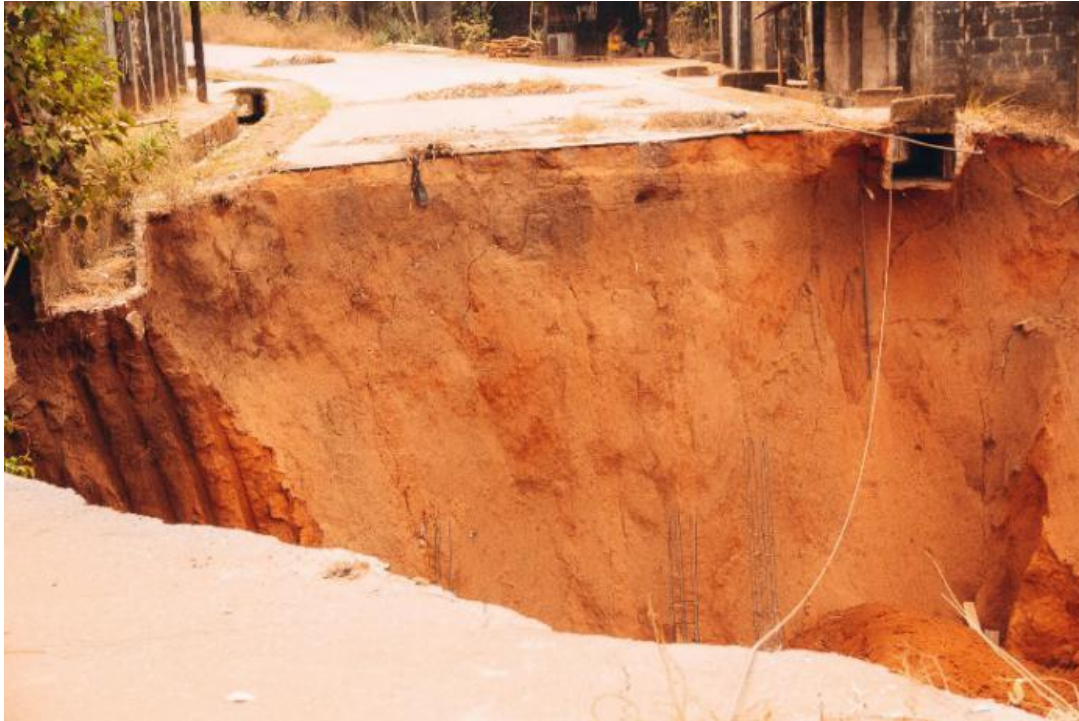
Fig. 3: Gully erosion site at Ezinifite Road, Ebenator
