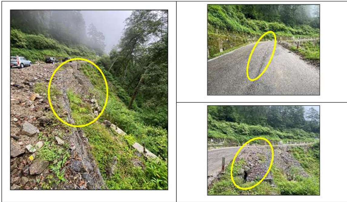
Fig. 1. Pre-failure field evidence showing tension cracking and progressive valley-side distress at Km 19.80.
