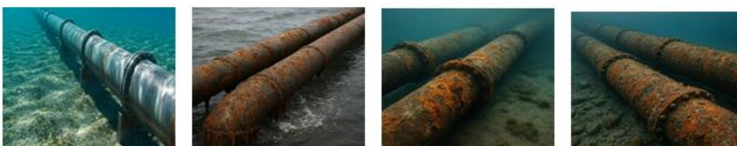
Figure 9(d): Representative normal and corroded marine pipeline image samples used for CNN-YOLOv8 training
