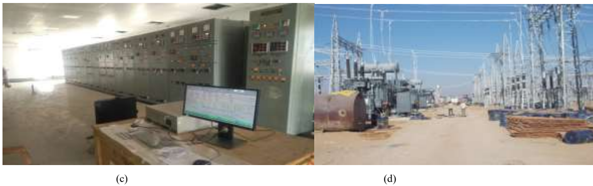
Figure 4 (a) Bhadla Phase II Solar Park (b) & (c) Control Room of Bhadla GSS (d) 400 kV Bhadla Substation
