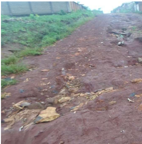
Figure 4: Degraded roads in Mbouda town.
