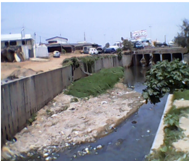
Fig.4a Siltation of Onyasia River at the confluence with Odaw River
