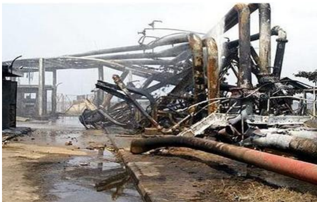
Fig 5: A vandalized oil pipeline
