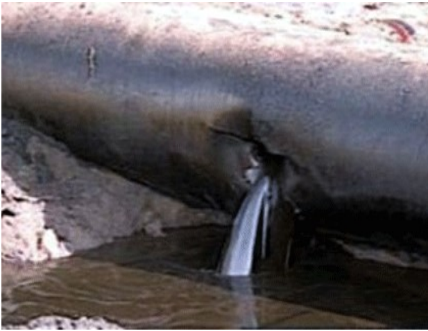
Fig 2: A vandalized Pipeline
