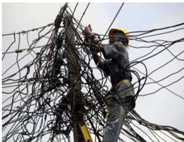
Fig 7: An example of existing electric wire and cable outlook. Source: (Victor Ahiuma-Young et al., 2017 & Olamide, 2017).
