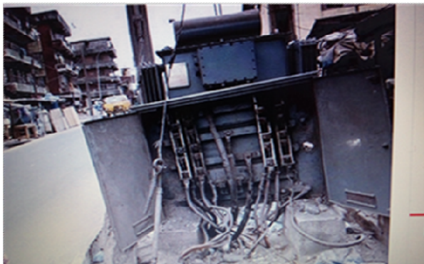
Fig. 4: Distribution Transformer current situation Source: (Occupational Safety and Health Administration, OSHA. 2017).
