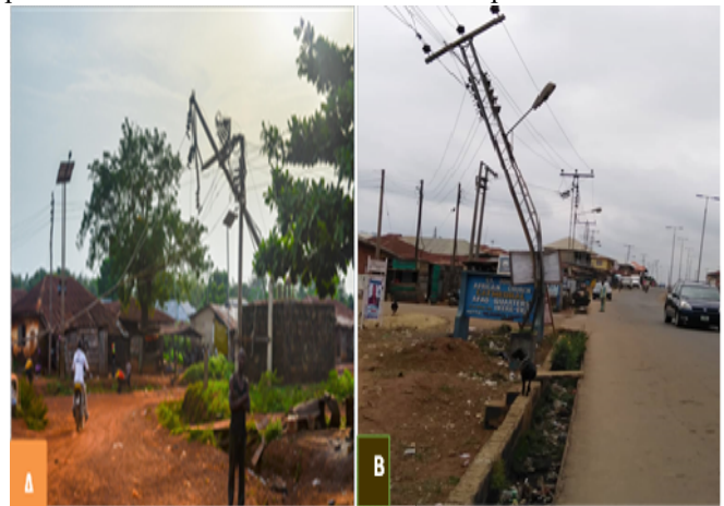
Fig 6: (A) Low tension electric poles condition, (B) Source: Author's fieldwork (2020) Source: (Abiodun, 2015 & Olamide, 2017)
