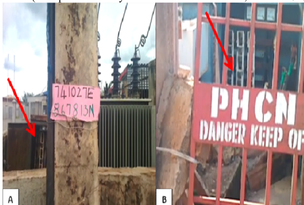
Fig 5: Overloaded distribution transformers in, (A) Ido Ekiti and (B) Ikole Ekiti Source: Author's fieldwork 2016
