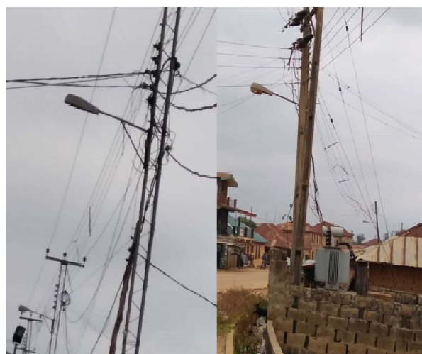
Fig 8: Uncoordinated warping electric wires with the bracing sticks, Source: Author's fieldwork
