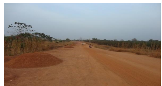
Figure 2. Anshagba-Ikyobo-Ge road under construction for over five years (January, 2017).
