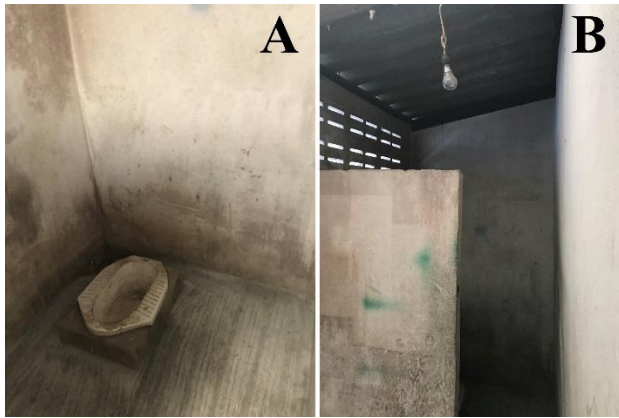
Figure 12: Bathroom with inadequate equipment (A) and low wall partitions (B) in Srinakarin, Bangkok (AR 4106, 2018)
