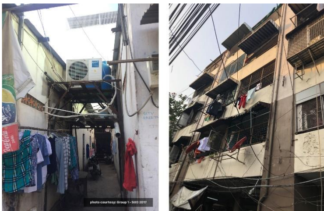
Figure 10: Messy electrical wires in Din Daeng Condominium, Bangkok (left) and Go Vap rental-room area, Ho Chi Minh City (right) (AR 4106, 2018 and SUD 2017, 2017)
