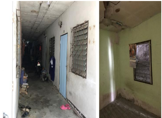
Figure 11: Poor lighting and aeration in the houses in Srinakarim, Bangkok (AR 4106, 2018)
