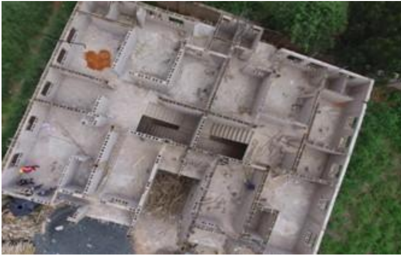
Fig. 5: Aerial View of an ongoing semi-detached duplex at WTC Estate. Captured by a DJI Phantom 3 Standard Drone.
