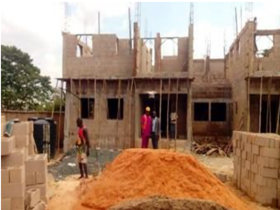
Fig. 4: Lintels being prepared on the upper floor; window openings and block work is visible for counting.
