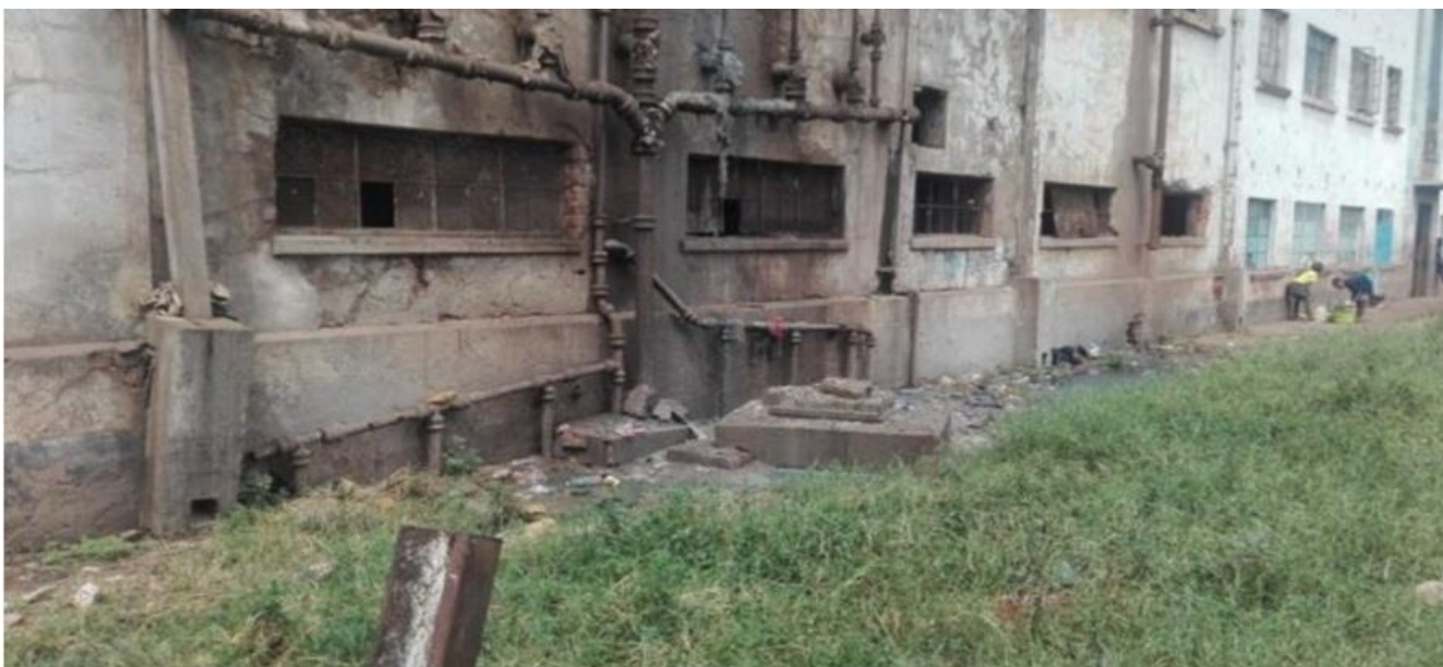
Photo 1: The state of sanitation infrastructure in one of the old suburbs of the Ancient city.
