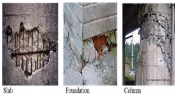
Fig. 3 Examples of Structural Defects
