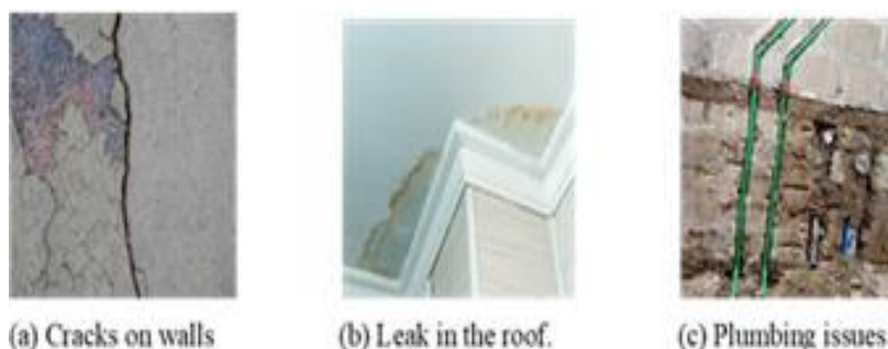
Fig. 2 Examples of Latent defects
