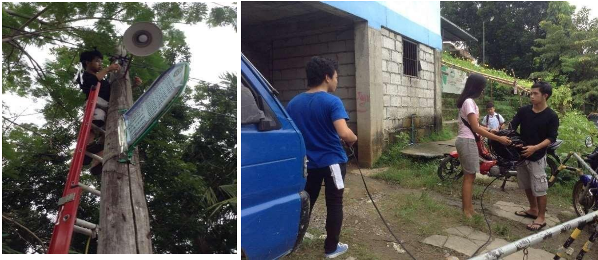
Figure 1. Actual installation of cameras within the vicinity of the Barangays
