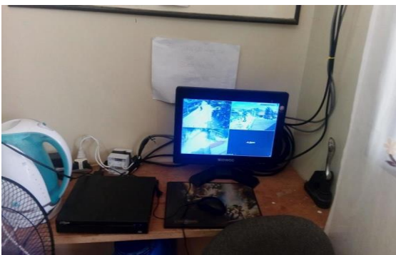
Figure 5. Display monitor of the areas under surveillance with the newly installed CCTV camera system for Barangay Tibig
