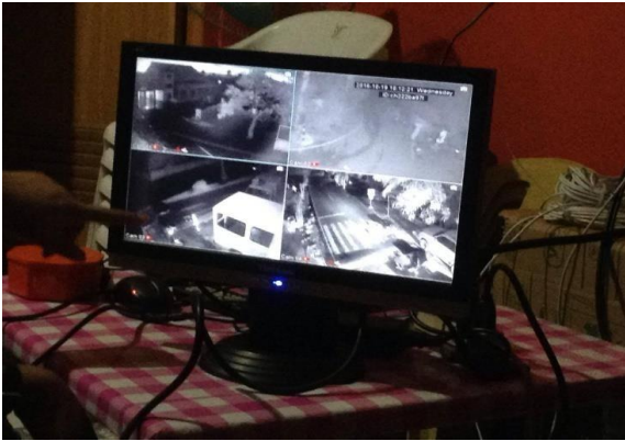
Figure 4. Display monitor of the areas under surveillance with the newly installed CCTV camera system for Barangay San Miguel
