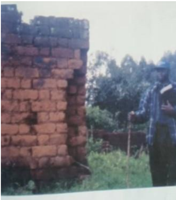
Plate 1: One of the Destroyed Houses in Yee
