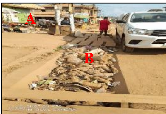
Photo 3: Blocked Drainage System in Mendong Coordinates: 3°53’34” N, 11°30’37”E Height above sea level: 730m
