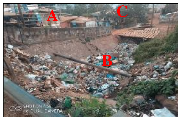
Photo 4: Blocked Drainage System in Simbock Coordinate: 3°53’34N, 11°30’41”E Height above sea level: 710m
