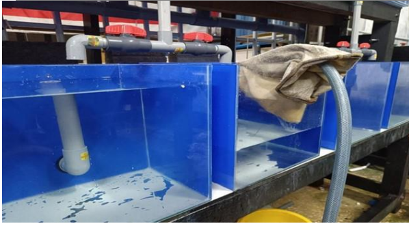
Fig. 3. Tank, marine water and treated freshwater
