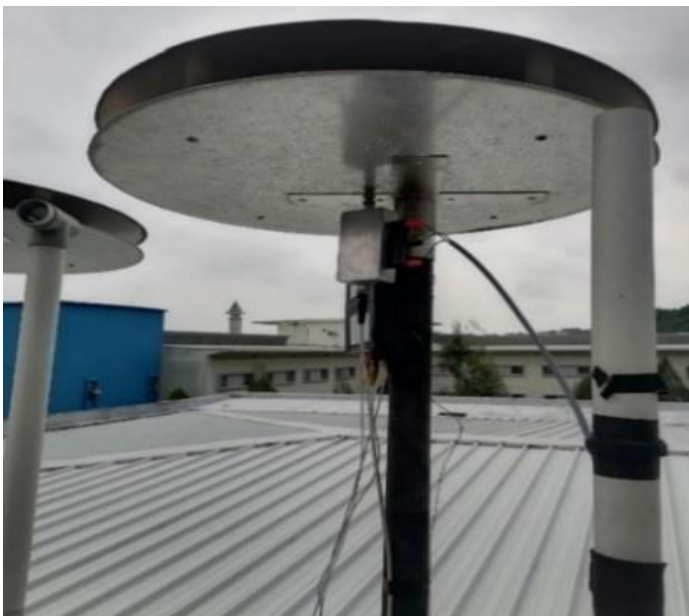
Figure 3. Installation setup for the lightning system in real time measurement
