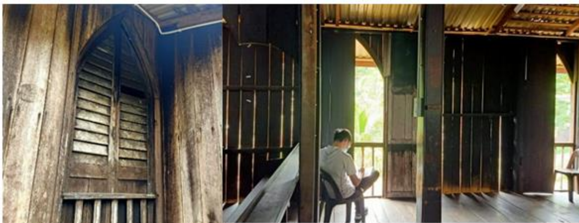
Fig. 13: Large timber louvers window opening for natural cross ventilation of St. James Church, Kampung Quop
