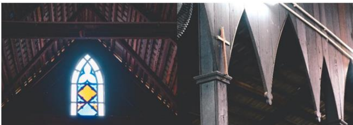
Fig. 10: High Clerestory Windows (Left) & Gothic Arches (Right) of St. James Church, Kampung Quop
