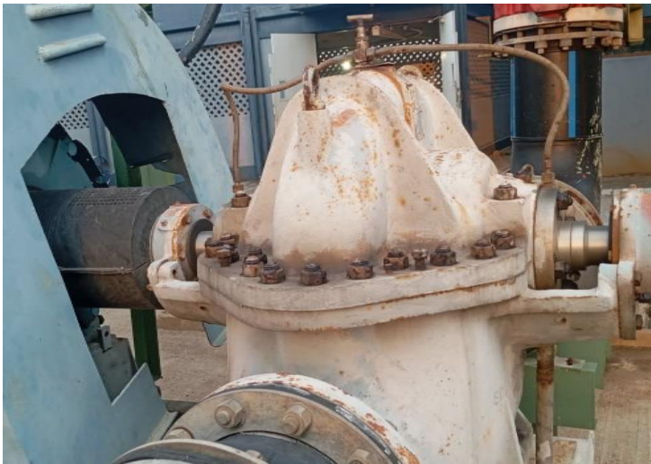
Fig 1. 50-P-007B UF backwash pump
