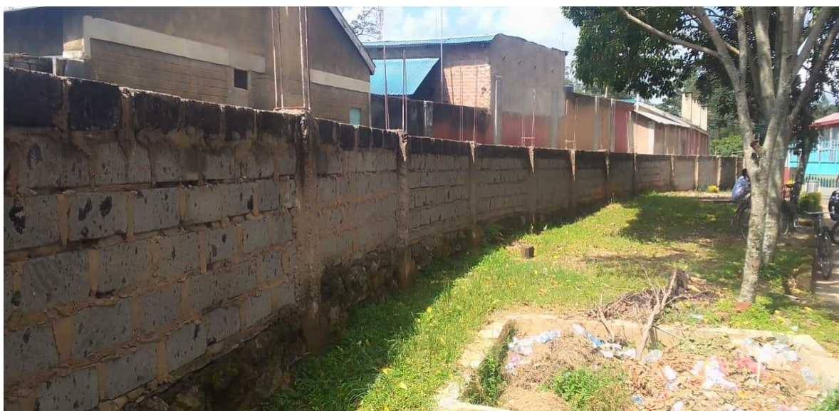
Stalled Perimeter wall of Institution B FY 2019/2020
