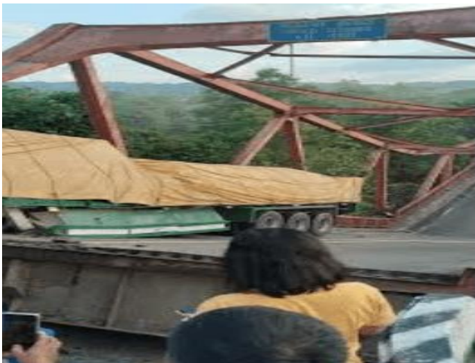
Photo # 13 - Broken Bridge
