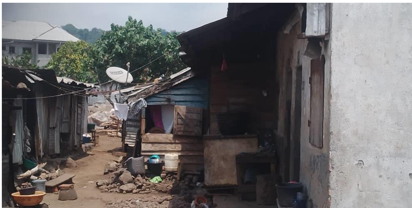
Figure 3: Dilapidated roofs of the CDC workers' camp at Likomba camp
