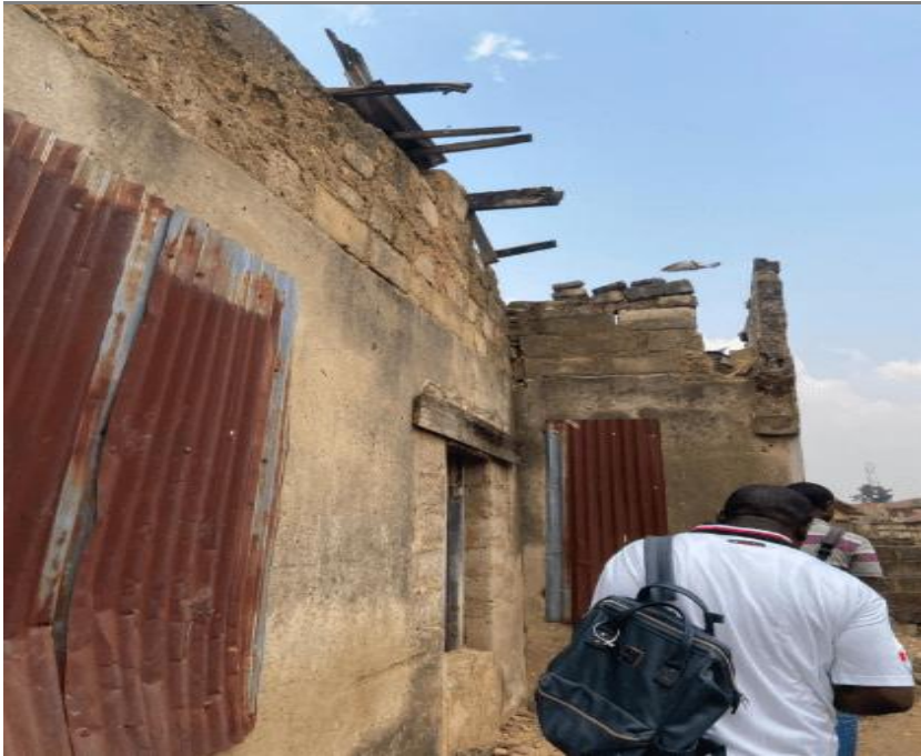
Fig. 4: Image showing the dilapidating condition of housing
