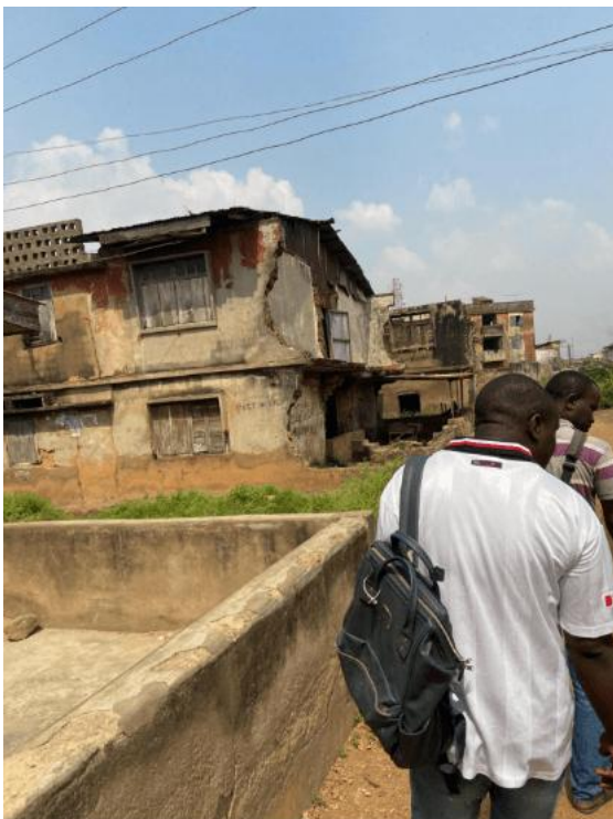
Fig. 5: Image showing the dilapidating condition of housing
