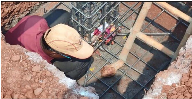
Fig. 5: Bhoomi pooja ceremony of house construction showing foundation deposit of note money, flowers, coconut, burning of incense, relics, ceramic utensils
