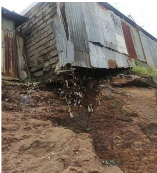
Figure 4: Illegally constructed house with poor foundation
