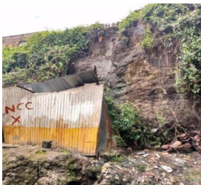
Figure 3: Illegal structure at the foot of a cliff fallen on by an avalanche during landslide
