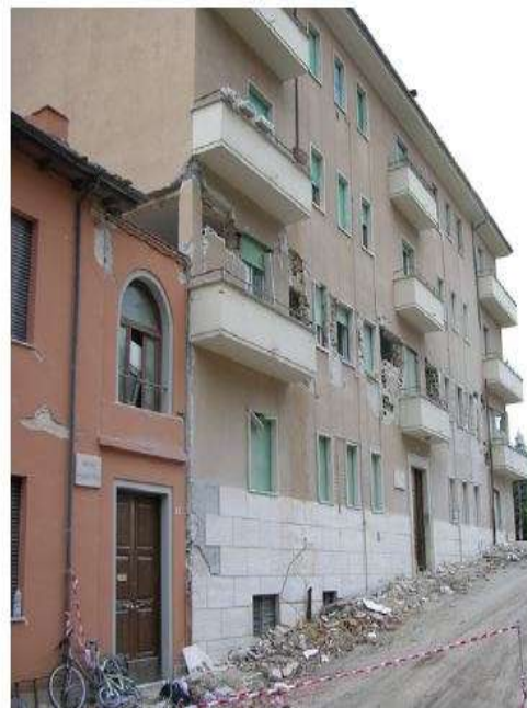
Fig 2: Damage of a four-story conventional building due to pounding with its adjacent two-story building, during the L'Aquila earthquake in Italy, in April 2009
