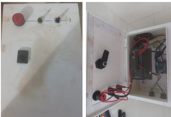
Fig. 5. Assembled electrical control cabinet for the integrated slotting mechanism
