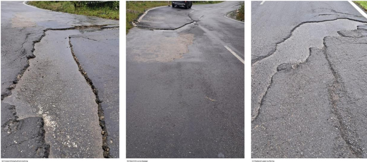
Fig. 1. Representative slippage/shoving distress in the loaded downhill lane, Km 40-72.8.
