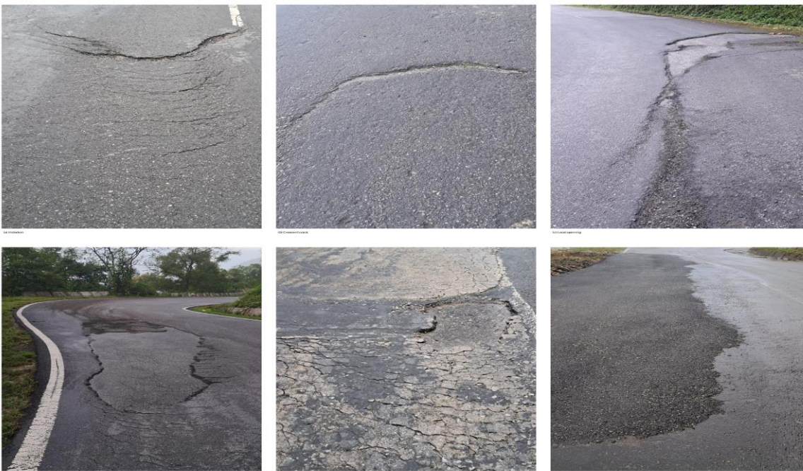
Fig. 2. Field-observed progression from crack initiation to advanced slippage and patch repair.
