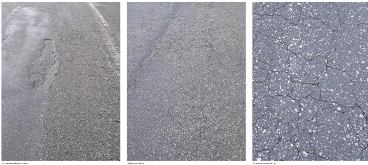
Fig. 3. Representative cracking distress in Km 5-40.
